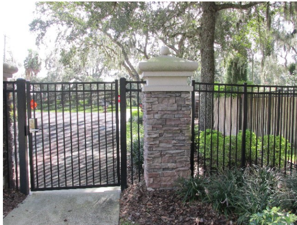
Leaning pillar due to tree roots
