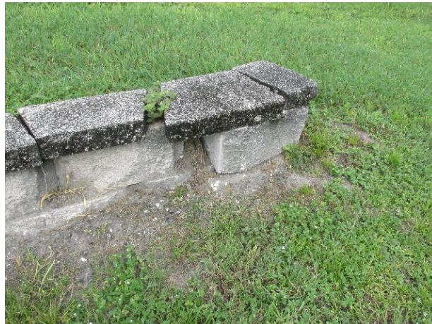
Shifted blocks evident
