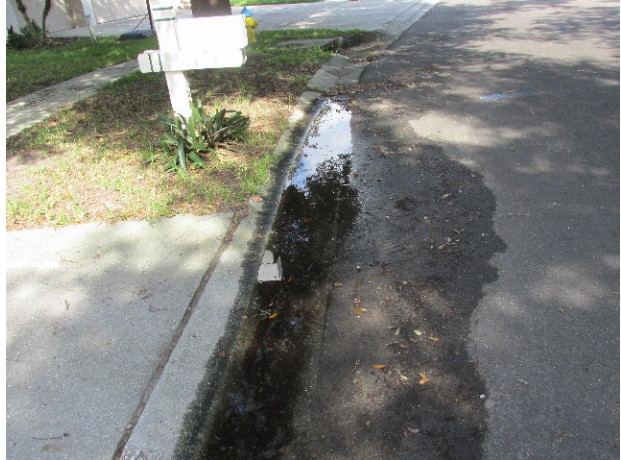
Standing water evident
