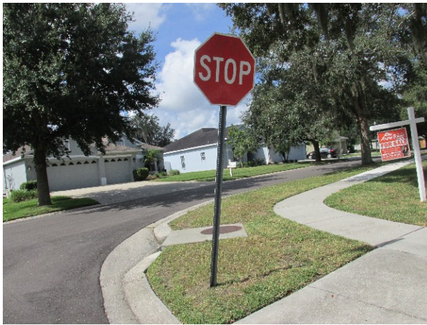
Leaning stop sign
