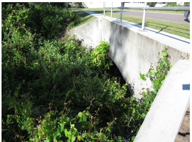
Box culvert with overgrown vegetation
