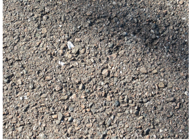
Asphalt pavement with raveling
