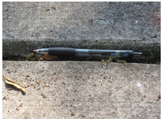
Sidewalk with trip hazard
