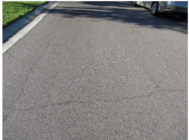
Asphalt pavement with block cracks
