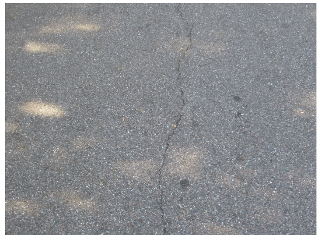
Asphalt pavement with longitudinal cracks
