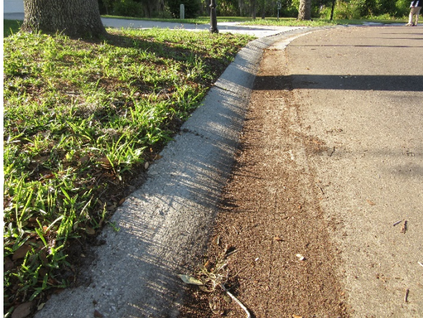
Concrete curb with evidence of water pooling on Moss Island Drive
