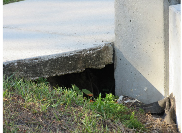
Gap between the sidewalk and box culvert on Moss Island Drive
