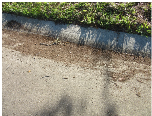
Concrete curb with evidence of water pooling on Moss Island Drive
