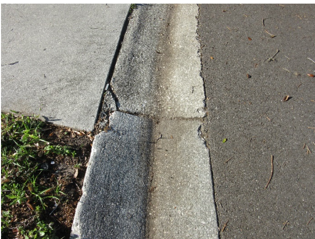
Concrete curb with cracks evident
