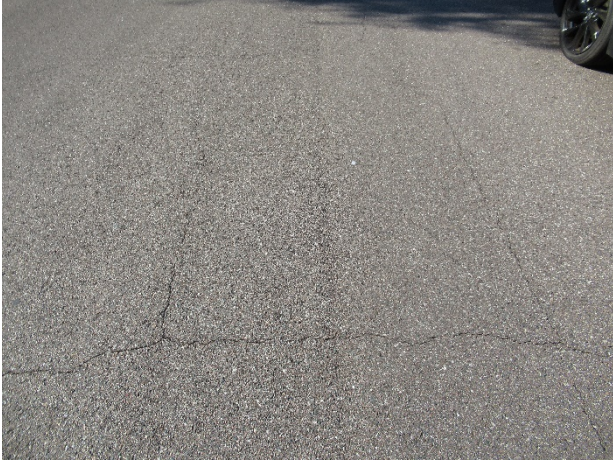
Asphalt pavement with block cracks
