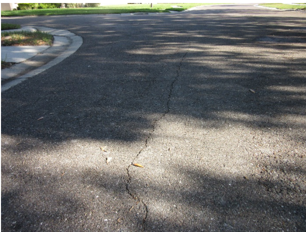
Asphalt pavement with longitudinal cracks
