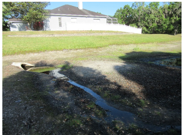
Bridgecreek Drive pond with soil accumulation evident
