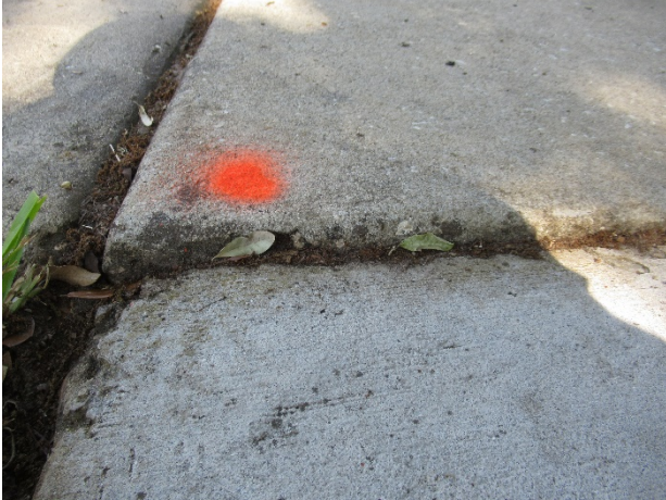
Sidewalk indicating trip hazard location
