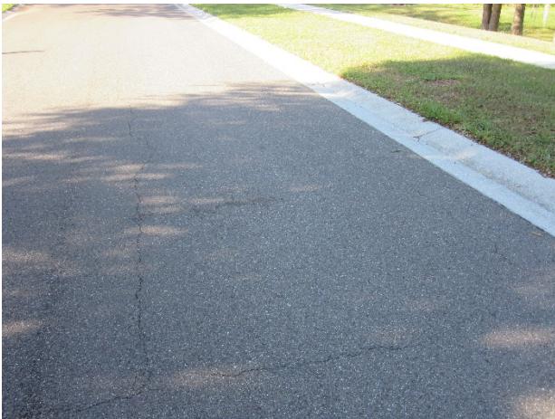
Asphalt pavement with block cracks on Moss Island Drive
