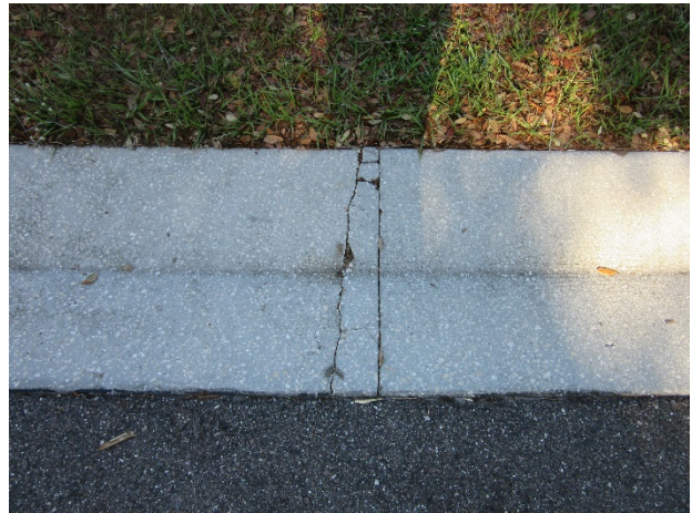
Concrete curb with common cracks
