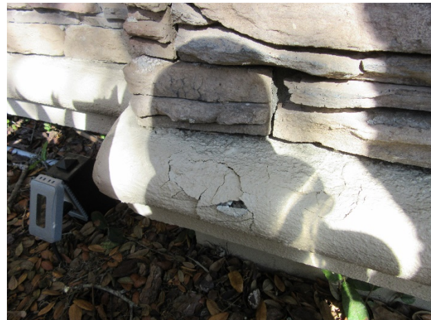
Architectural foam damage on front entrance pillars
