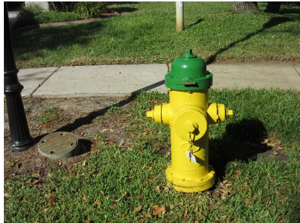
Fire hydrant maintained by Hillsborough County
