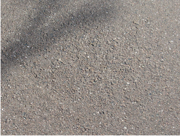
Asphalt pavement with mild raveling
