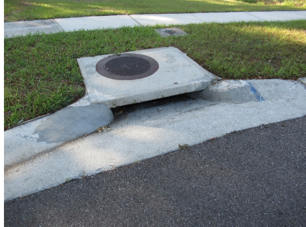
Catch basin with signs of repairs
