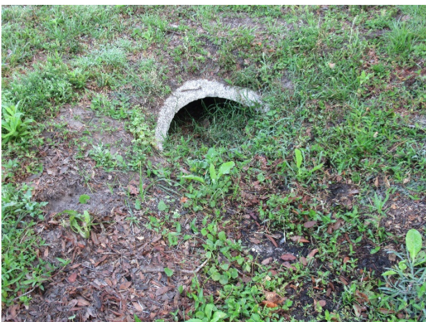
Pond outflow pipe with sediment accumulation
