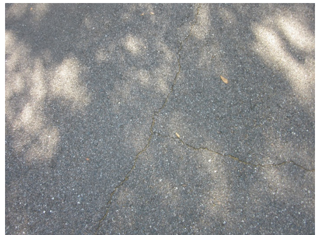
Asphalt pavement with longitudinal and Transverse cracks
