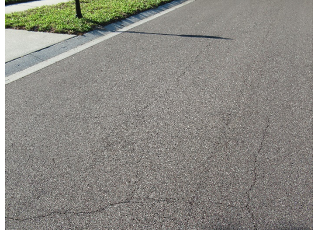
Asphalt pavement with block cracks
