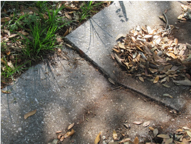
Lifted concrete curb
